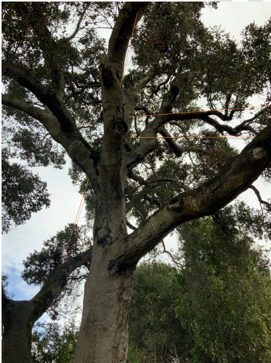
Four of the 7 cables highlighted in orange. Position of highlight is purposefully offset of position of cable for reference.
